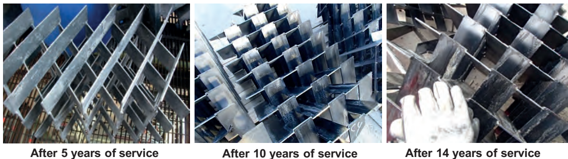
Figure 2 Stripper packing inspection images
